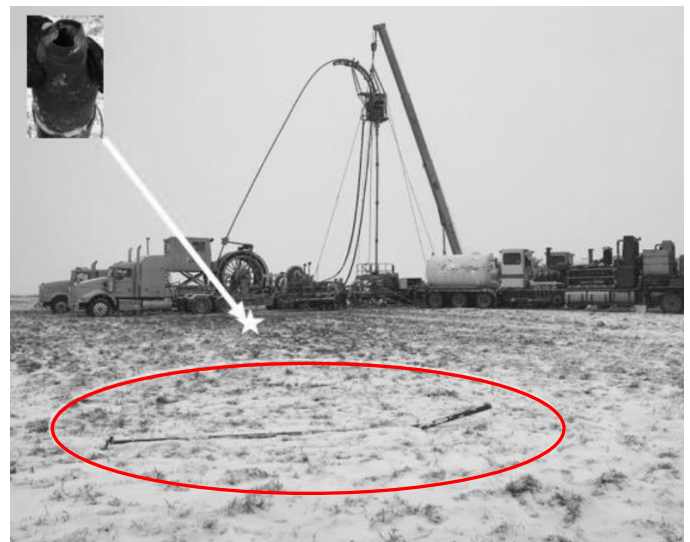
View of where blowback piping (red circle) and fitting (white arrow and star) landed on south side of site.
