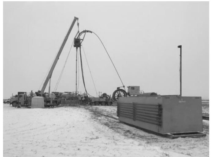
View of blowback piping and tank on the north side of site prior to overpressure event.
