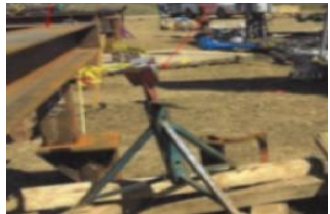
Example of unstable pipe stand
