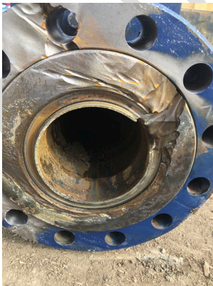
Figure 26. Example Flange Failure
