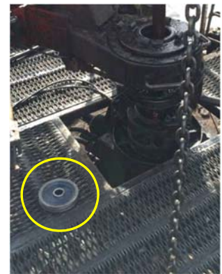
Sheave that fell to rig floor
