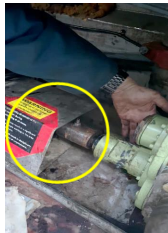
Pump shaft with the guard that is normally in place
