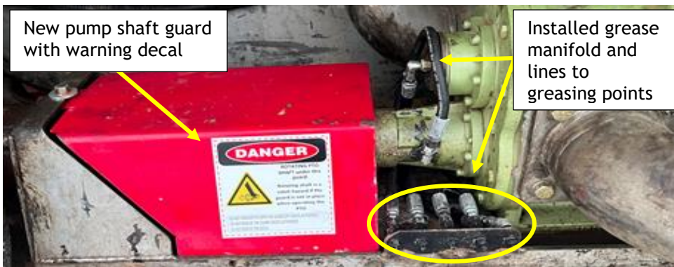
View of modified guard and grease manifold
