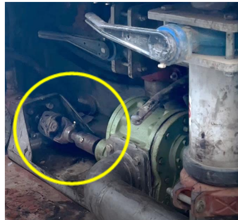
View of the exposed pump shaft with no guard
