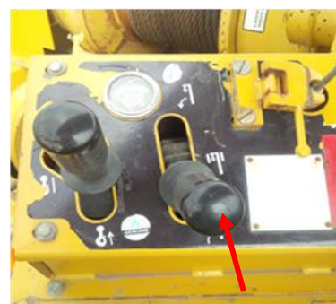
The boom stick control lever stuck in the engaged position.
