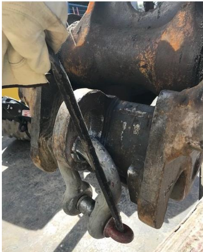
WORKER HOLDING THE PIN BAR ON A SHACKLE AT THE BACK OF AN EXCAVATOR
