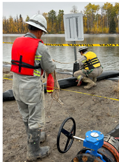
Example of personnel working as a team using life jackets and utilizing fall restraints.
